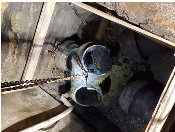
16 inch Wye removed from 1880's cast iron main at Central and Main Street
