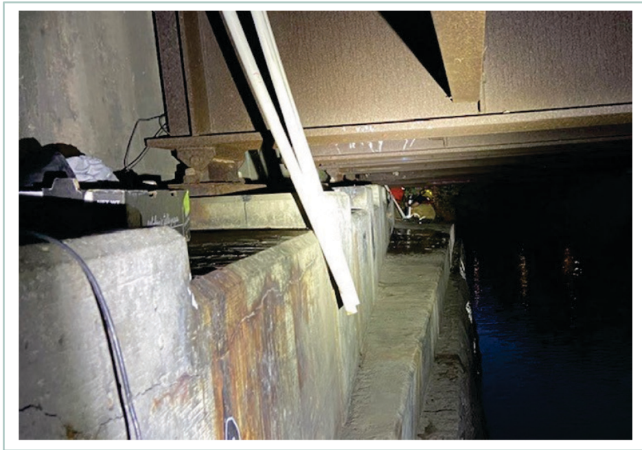
Crews on their stomachs at the far end of the bridge abutment, evaluating the fire under the bridge.
