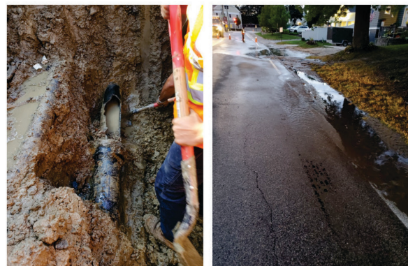
Hough Street leak prior to being turned off.
