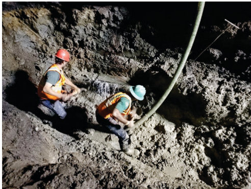
Lateral Main break on Oak Street.
