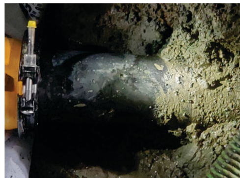
2 nd leak on Oak Street.
