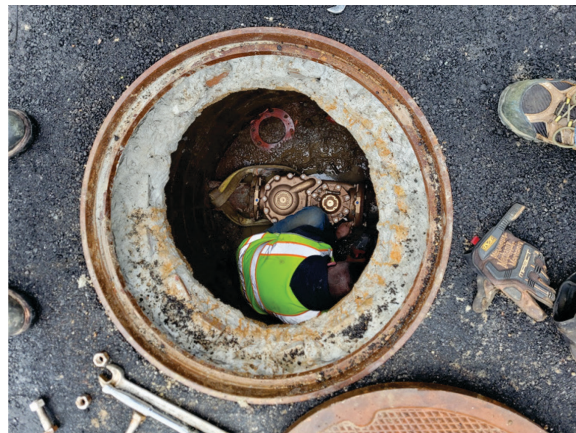
Union Street new compound meter in the vault.
