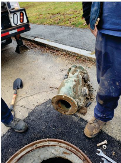
Union Street old compound meter.
