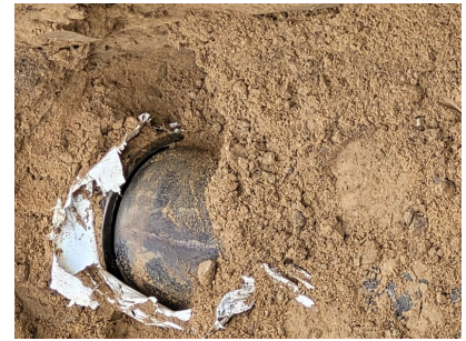
Water main separated at Spur Road
