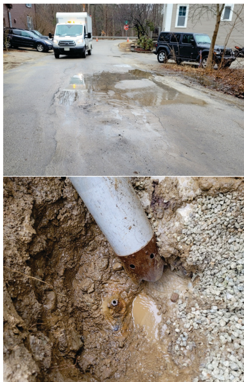
Leak on Snows Court
