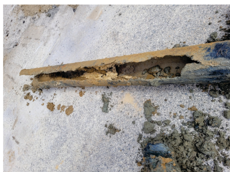
Damaged Sewer Main Hampshire Circle
