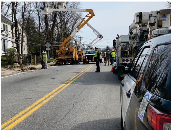
Lieutenant Marn Speidel and utility crews from Eversource survey the damage to a pole at 151 Central Avenue.
