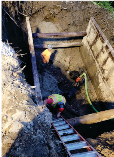
Water mains have been cut out.
