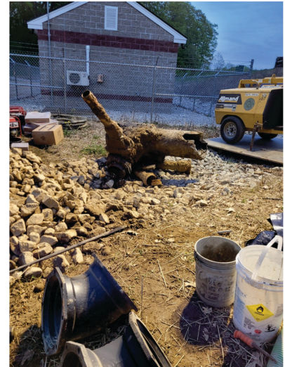
Tee & A/C water main.
