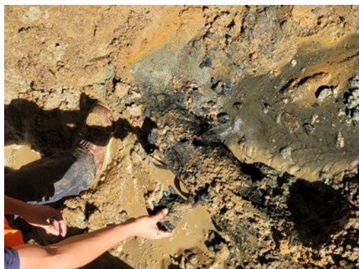
Hough Street rotted off saddle
