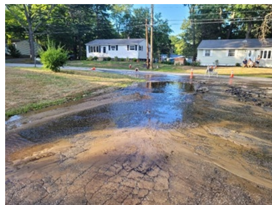
Tanglewood Water Main Break
