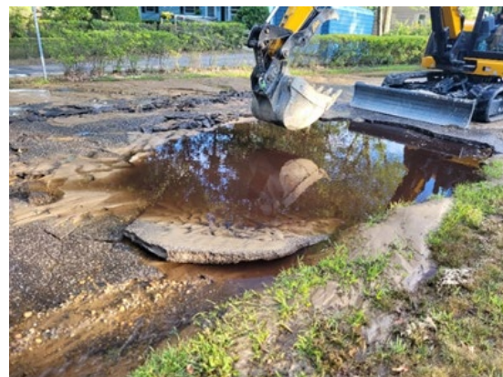
Tanglewood Water Main Break
