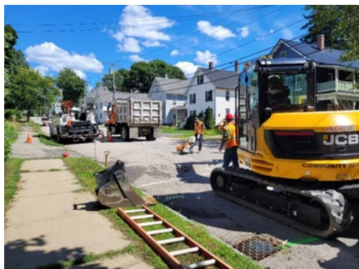
Hough Street Water Main Break
