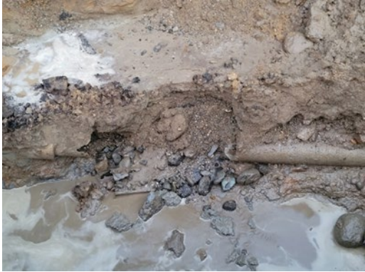
Tanglewood Water Main Pre-Repair
