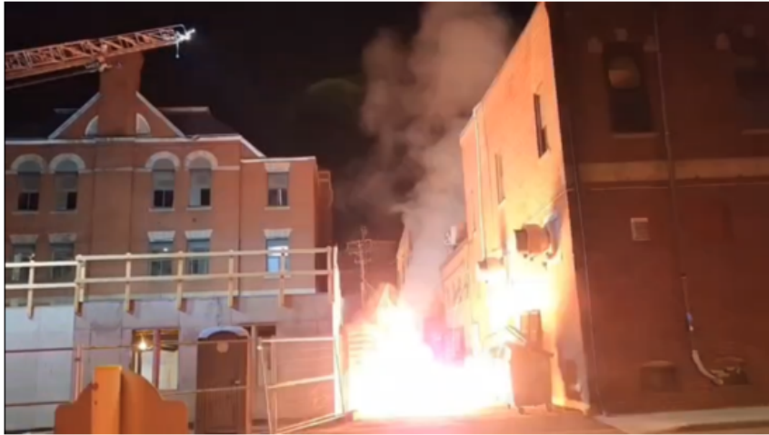
Photograph from First St. of the lower man-hole during one of the explosions from the underground high voltage electrical fire.
