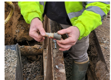
Cause of water leak on resident side of service
