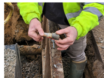
Cause of water leak on resident side of service
