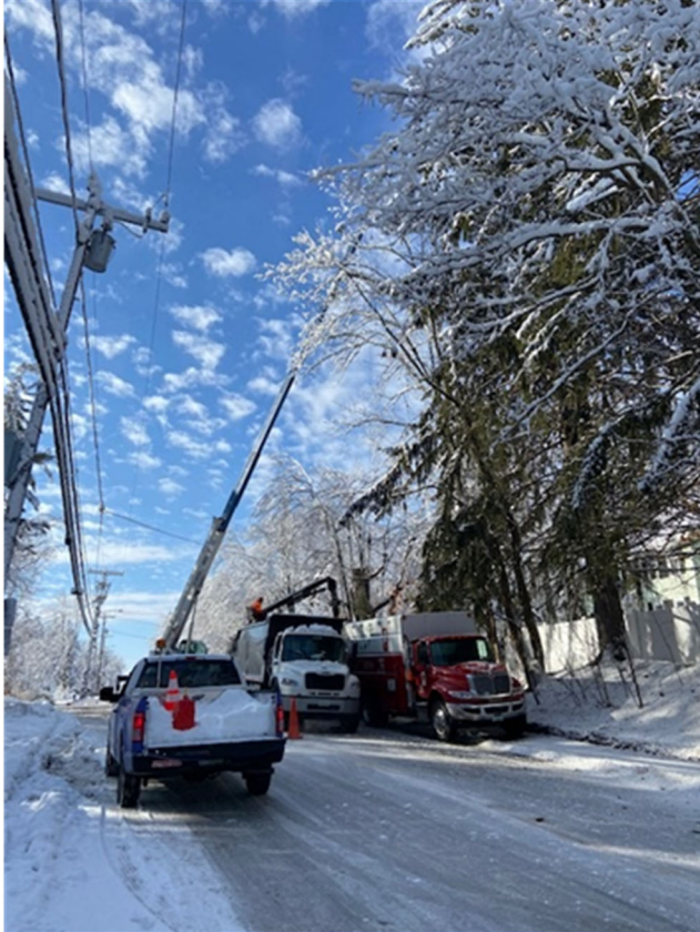
Crews work to remove an 80-foot-tall pine tree that was compromised as a result of the storm. The tree was damaged and about to fall across Durham Rd. and would have taken down a three-phase power supply on the Rt 108 corridor.
