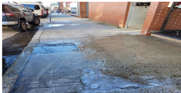
Asia restaurant fire line freeze up.
