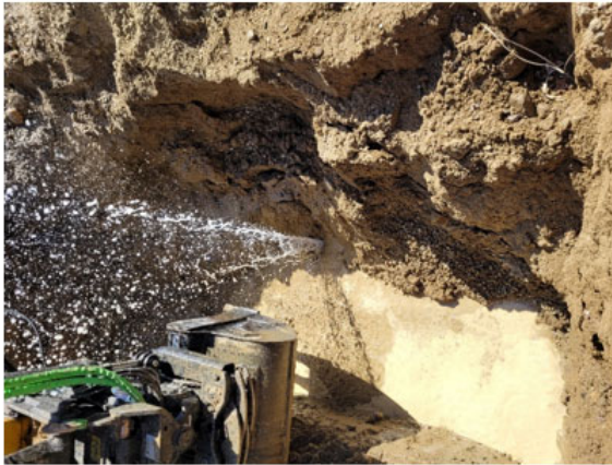
Above: Hole in main on Hough St
