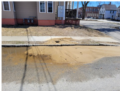
Above: 4 Grove St leak
