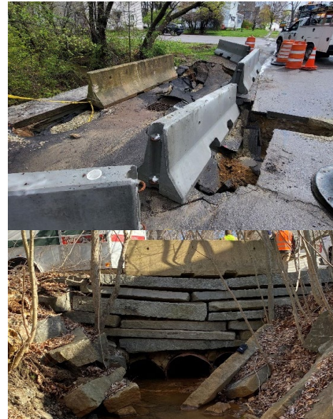
Figure 1: Failed triple culvert below Hough Street.
