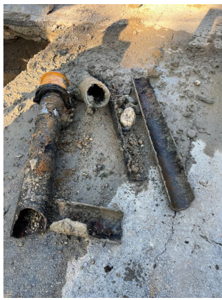
Hough Street water main failure.
