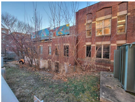
The trees and overgrowth were removed up against the building at the Children's Museum
