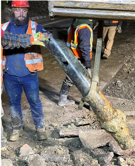
Broken Water Main Locust Street
