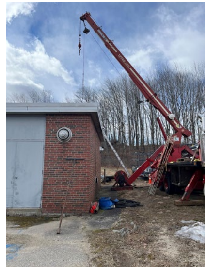
Griffin Well cleaning equipment
