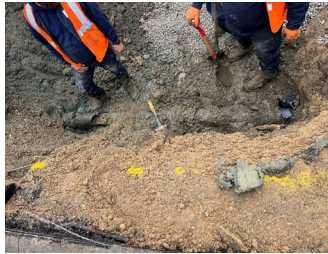
Rollins Road water main break
