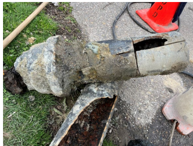
Oak Street water main break
