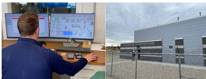
Seth Thompson of Community Services fires up the Pudding Hill Water Treatment Plant for the first time on May 2, 2024.
