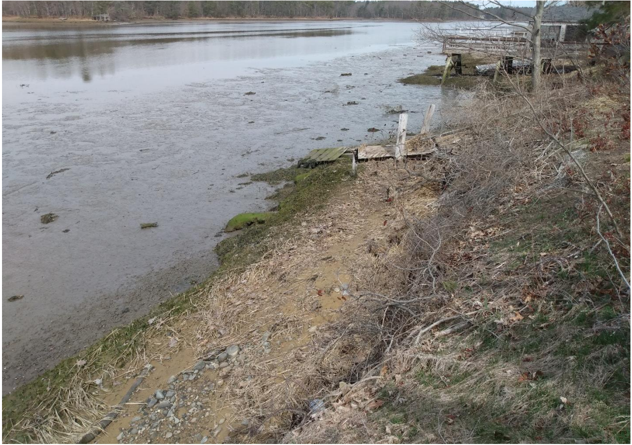
Photo 1 Site shoreline overview and collapsed dock. By CNE on 4-11-23
