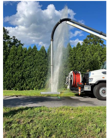
Force Main under pressure.
