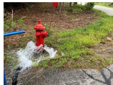
Hit hydrant on Willow St.
