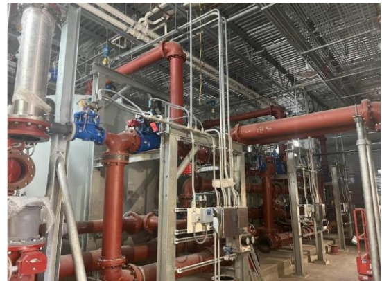
Interior of the new Pudding Hill Water Treatment Plant that treats upwards of 1 MGD of drinking water.
