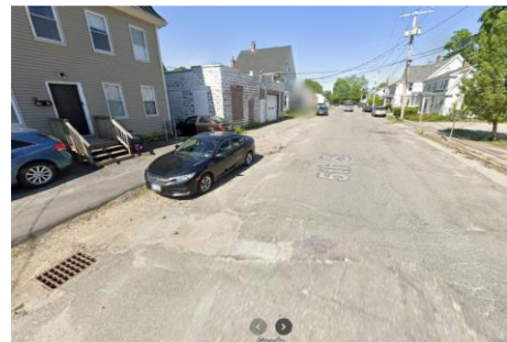
Fifth Street Deterioration in May 2023 prior to reconstruction (via Google).
