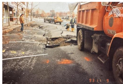
Water main break in Central Ave near Second Street from November 9, 1993.
