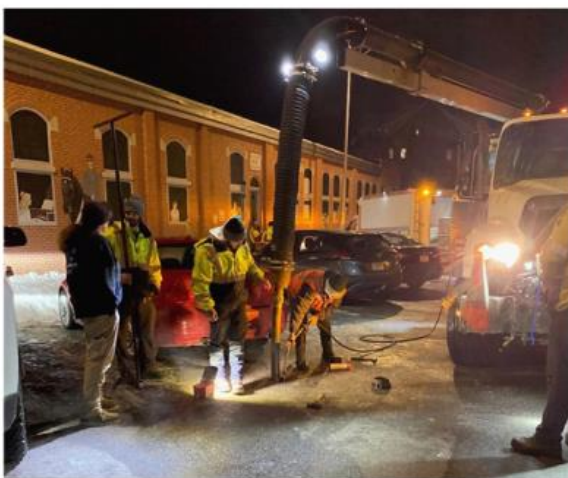
CS crews vacuum out a water shut off in front of the former Earcraft music building during the hunt for a water leak on February 8th.
