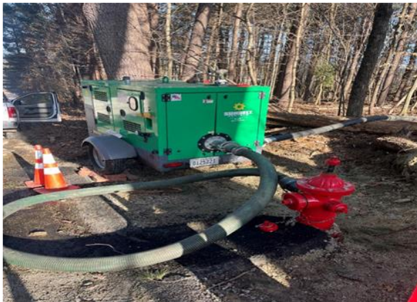
Pump used to drain Garrison Tank.
