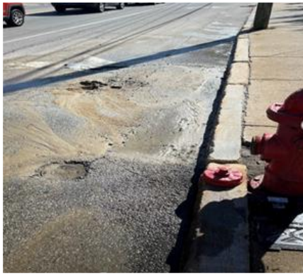
Broken valve on Central Ave by Silver St
