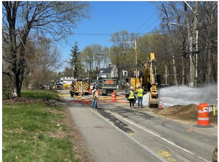
Representatives from Unitil assess the gas leak in Durham. Master stream is used to dissipate the leaking natural gas.
