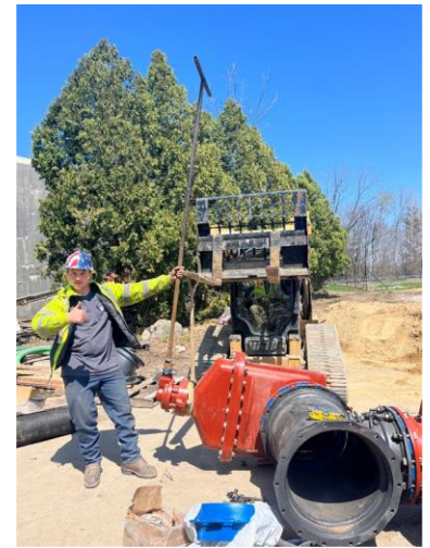
New valve assembly at Garrison Tank.
