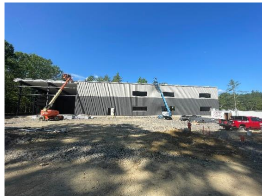
Future Automation Quality Way
