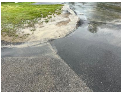
Water main break on Oak Terrace.
