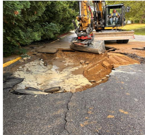
Olde English Village water main break
