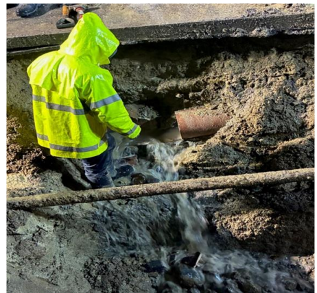
Broken drain line and old gas line encountered prior to locating the water main on Mount Vernon St
