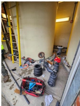
Double walled piping installed for Sodium Hypochlorite.
