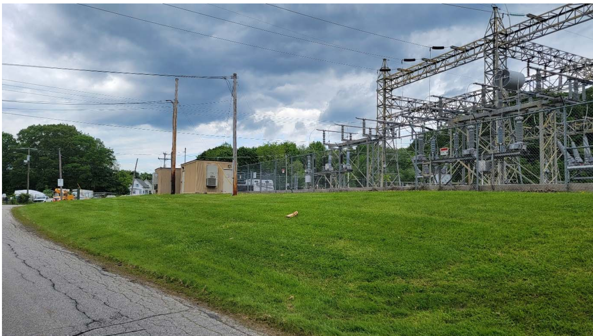
Photograph No. 6: Looking northwest from Cocheco Street at the existing substation.
