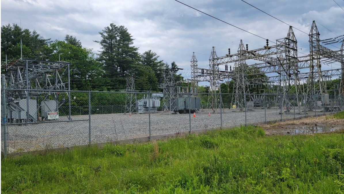
Photograph No. 3: Looking southeast at the existing substation infrastructure.
