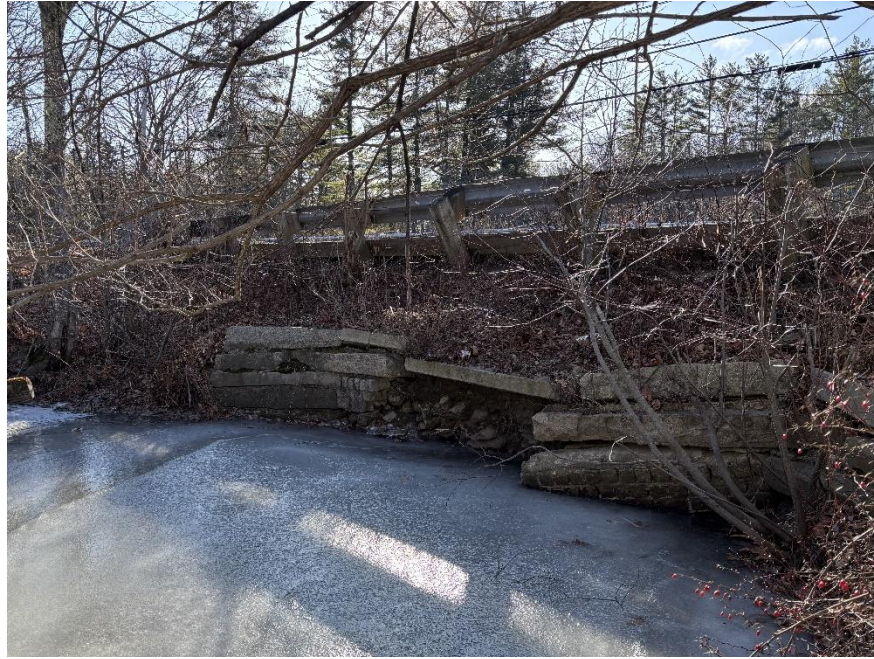
Photo 1 – Inlet of Granite Box Culvert in Unnamed Stream at County Farm Rd Blocked w/ Debris
