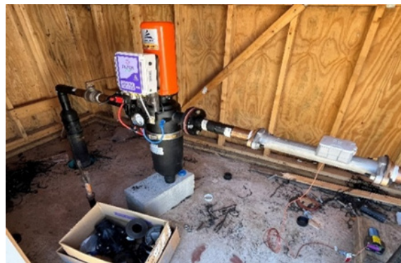
New pump system.
