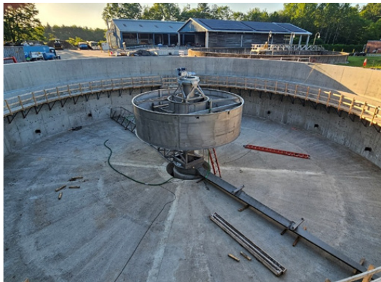
Install of Clarifier Mechanism.
