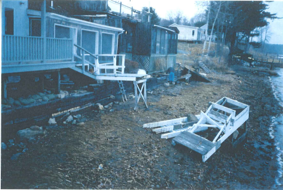
PHOTO #1: LOOKING NORTH AT EXISTING PIER DAMAGED DOCK AFTER FLOOD APRIL 2007
