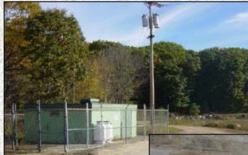
Ireland Production Well
