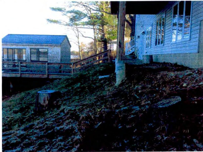
PHOTO 2: View looking northwesterly along the back side of the property. The permeable patio is required to level and stabilize the footings of the existing deck. Native plantings will be installed just down gradient of the patio in the existing lawn to enhance the buffering capacity and habitat value of the shoreline.
