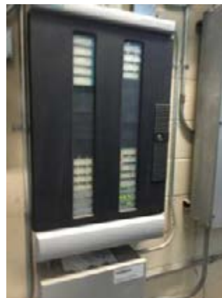
Existing High School Boiler Room ATC DDC Control Panel
