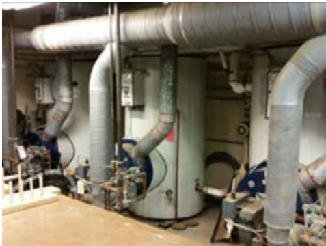
Original building water heaters
