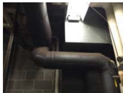
Interior Boiler Breeching
