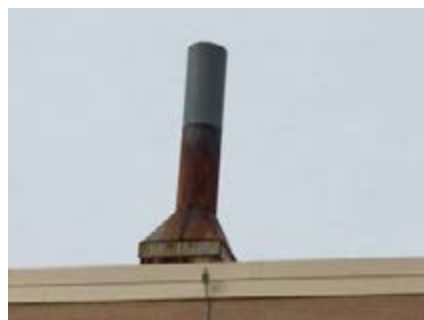
Exterior Boiler Breeching Stack
