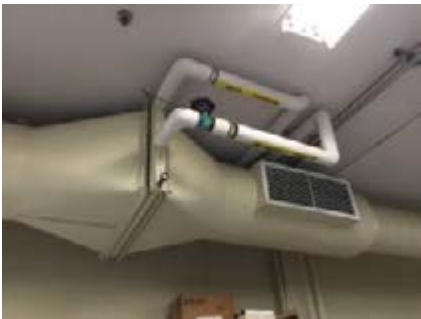
CADD Shop Heating Coil and Ventilation Ductwork
