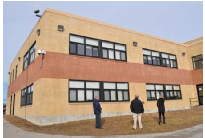
2002 Addition with Visible Efflorescence
