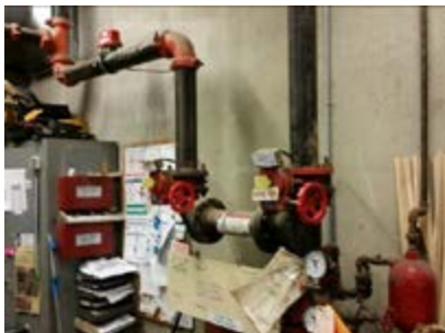
Fire service riser
