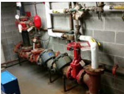
Combined water service - FP riser
