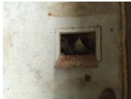
Auto Shop Under Slab Exhaust
