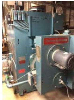
Existing Boiler (CB Burner)
