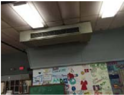
Music Classroom – Unit Ventilator
