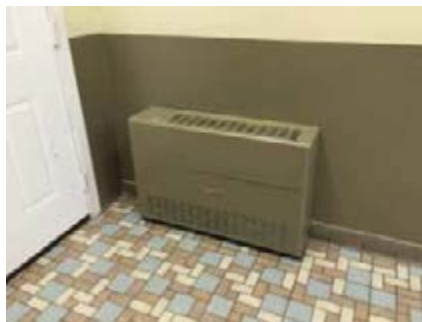
Existing Cabinet Unit Heater
