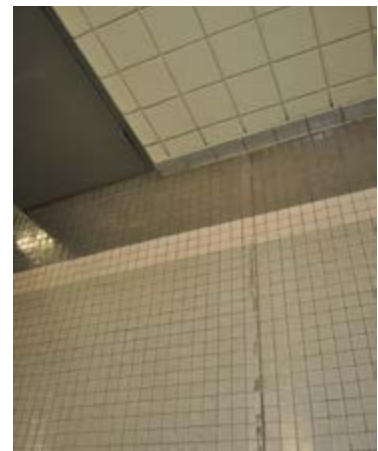
Cracked Tile Floor
