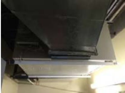
Administration Air Handling Unit
