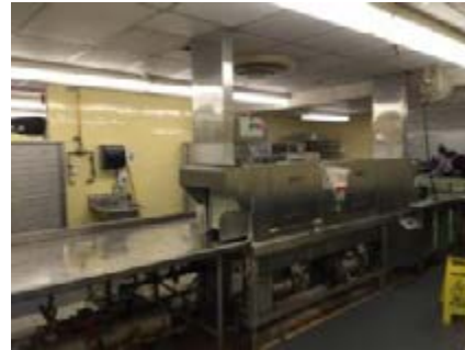
Dishwasher Exhaust Ductwork
