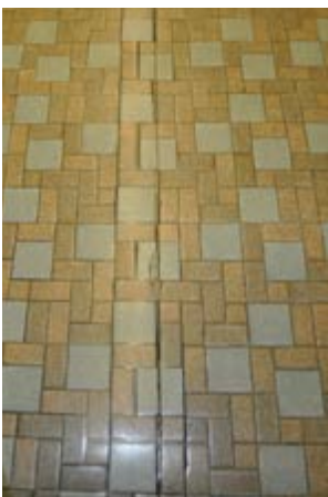
Cracked Tile Floor
