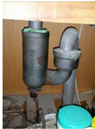
Science waste piping
