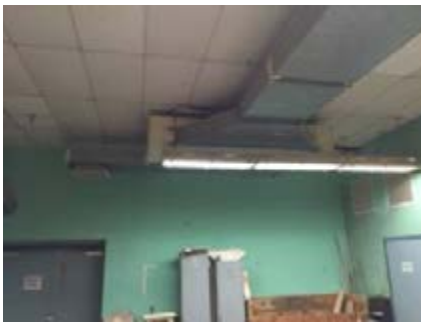
Wood Shop Unit Ventilator
