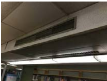
Library Heating & Ventilation Unit
