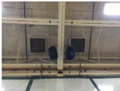
Gym Exhaust Grille
