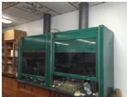
Science Classroom Fume Hoods
