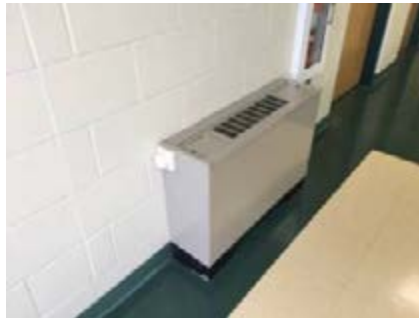
Existing Cabinet Unit Heater – World Arts Wing
