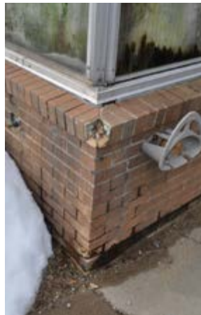
CTC Entrance & Brick in Disrepair
