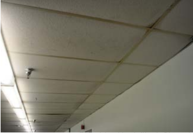
Typical Corridor Ceiling in Disrepair
