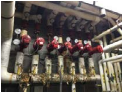
Existing Hot Water Pumps
