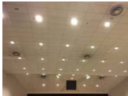
Auditorium - Ceiling Supply Diffusers
