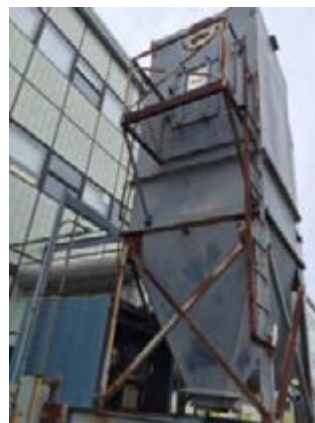
Wood Shop - Dust Collector
