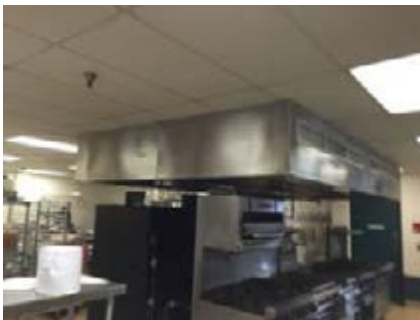
Kitchen Exhaust Hood
