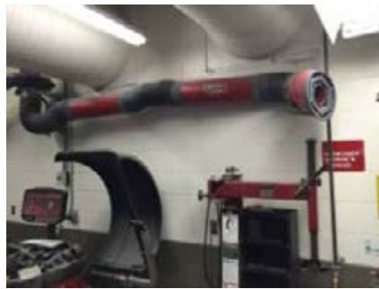
Auto Shop Welding Exhaust System
