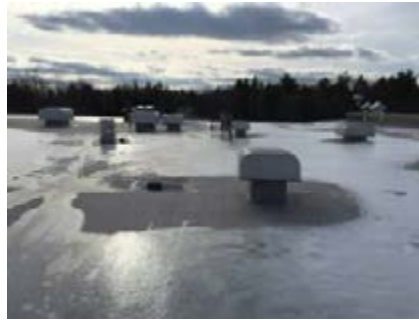
Roof Intake and Exhaust Air Hoods and Fans
