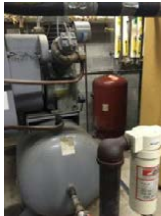
Existing Expansion Tank (back)
