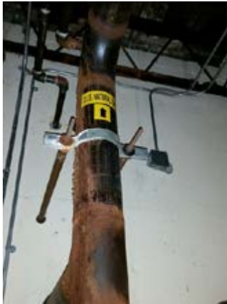
Original building gas piping
