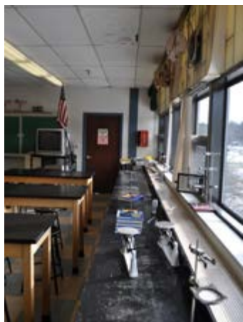
Counter Tops in Disrepair
