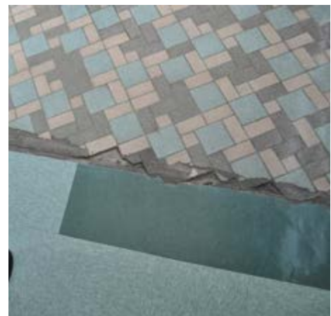
Missing Expansion Joint at 2002 Addition
