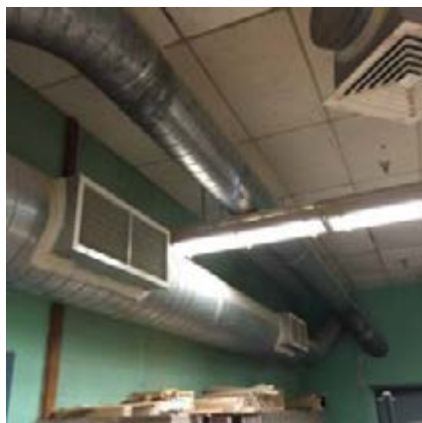
Wood Shop - Ventilation Ductwork
