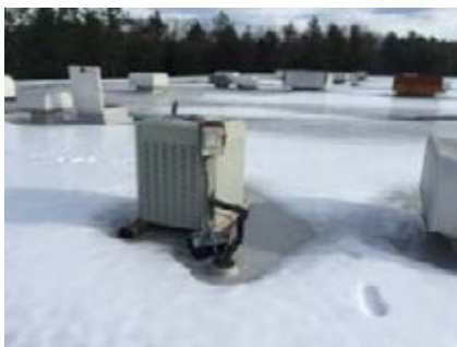
Roof ACC Unit
