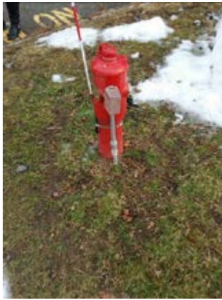
Post indicating valve
