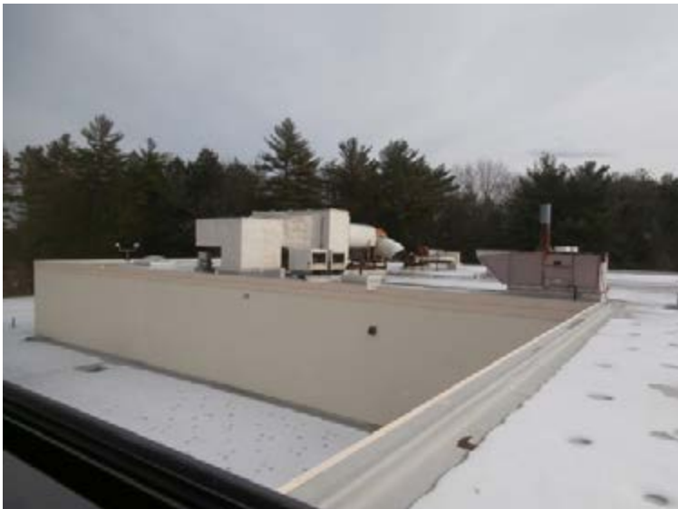
10. High and low roof areas of the 2002 CTC addition, looking NE from the third floor of the 1966 classroom wing.
