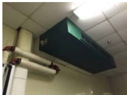
Locker Room Unit Ventilator
