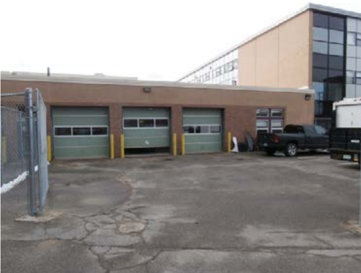
4. Low roof area, north side of 1989 addition, adjacent to three-story 1966 classroom wing.
