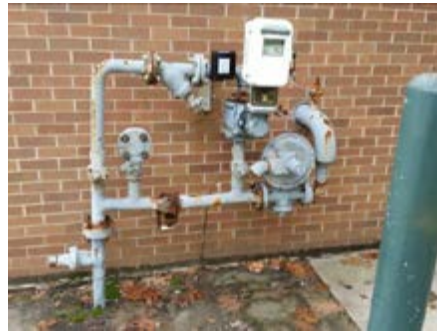
1987 building gas service & meter
