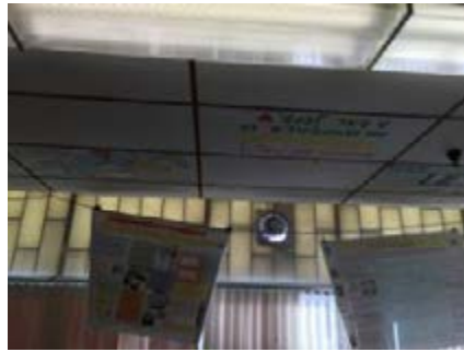
Science Classroom Sidewall Exhaust Fan
