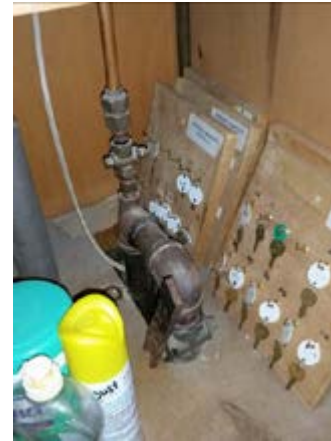
Science room gas valve
