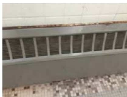
Locker Room Fin tube Radiation
