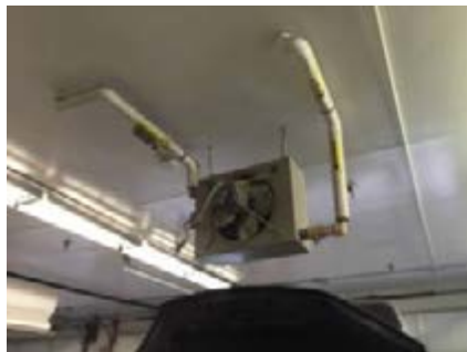
Auto Shop Unit Heater
