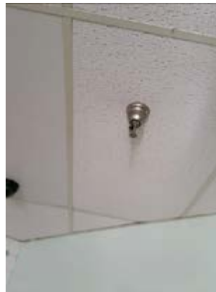
Typical pendent sprinkler
