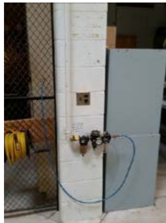
Typical air outlet station
