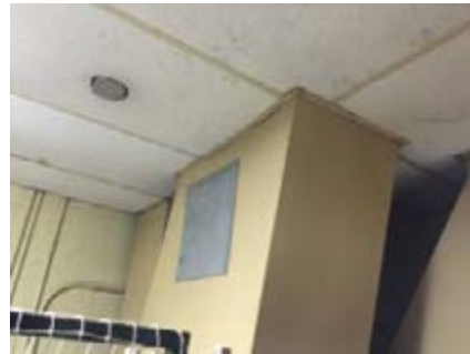
Kitchen Exhaust Duct Riser in Storage Closet
