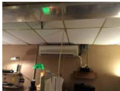
Ductless Cooling Unit – IT Server and Office
