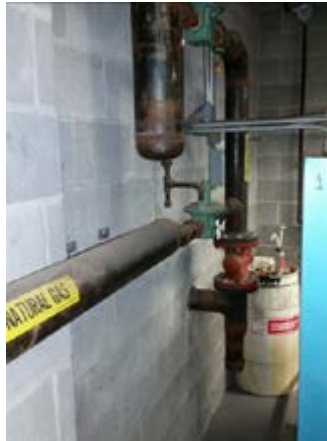
1987 building gas piping
