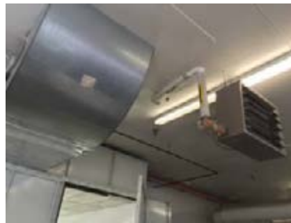
Paint Booth Ductwork and Unit Heater
