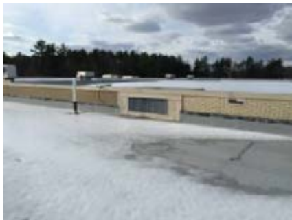
Unit Ventilator Intake Louver
