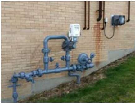
Original building gas service & meter
