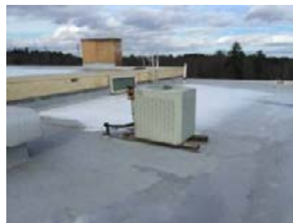
Roof ACC Unit
