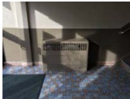
Existing Cabinet Unit Heater
