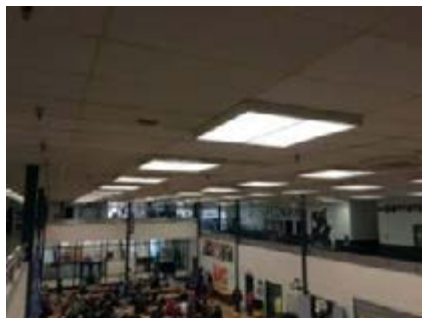
Cafeteria – Ceiling Diffusers
