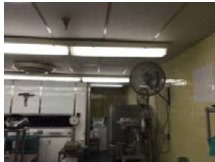
Supply Diffusers (left) and Prop Fan (right)
