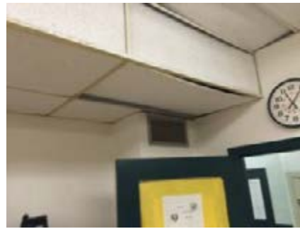
Classroom –Exhaust Grille
