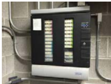
Existing CTC Building ATC DDC Control Panel
