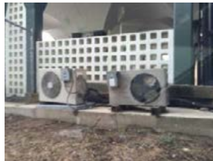
Ductless AC Unit ACC Units
