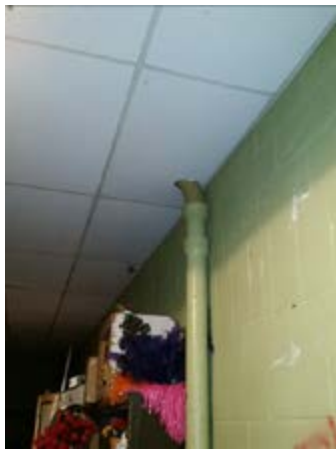
Cast iron drainage piping
