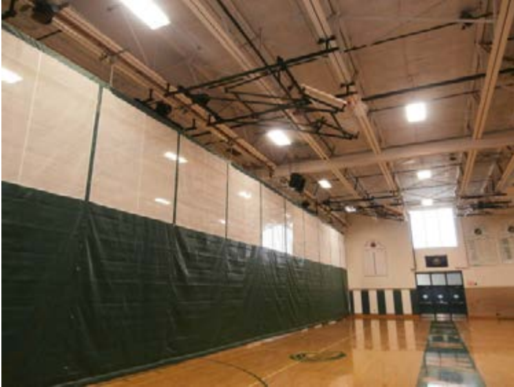
7. Gymnasium, long span open web joists, tectum roof deck on bulb tees.
