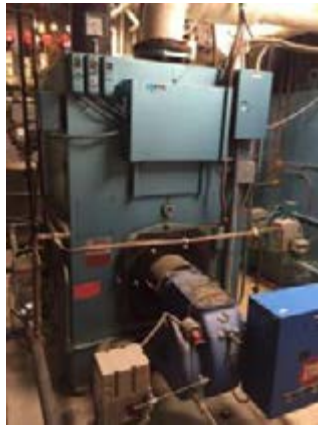
Existing Boiler (Johnson Burner)
