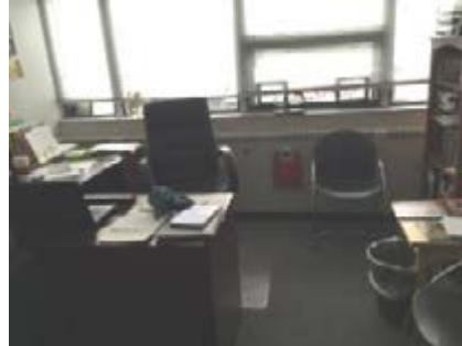
Administration Office – Fin tube Radiation Heating
