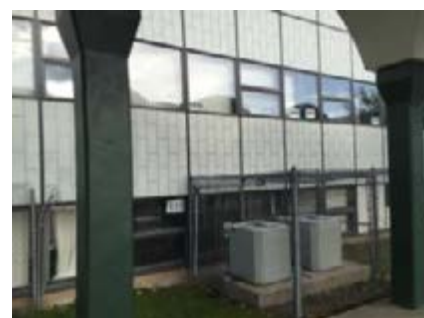
Grade Mounted Air cooled Condensing Units
