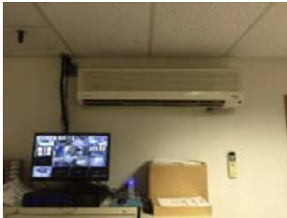
Ductless Cooling Unit – Operations Office
