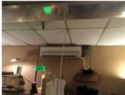
IT Room - Ductless AC Unit
