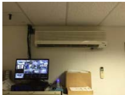
Administration Ductless AC Unit
