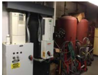
Existing HW Pump VFDs (left) and Expansion Tanks (right)
