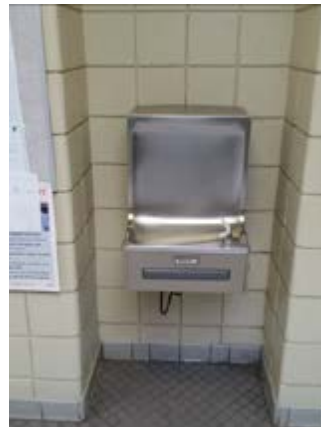
Electric water cooler
