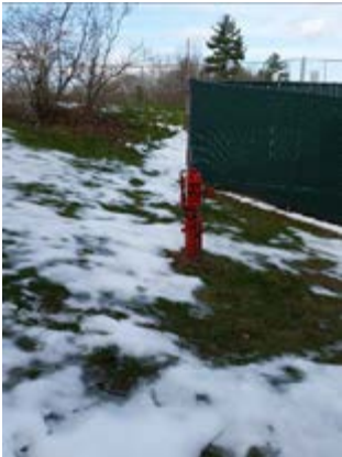
Post Indicating valve
