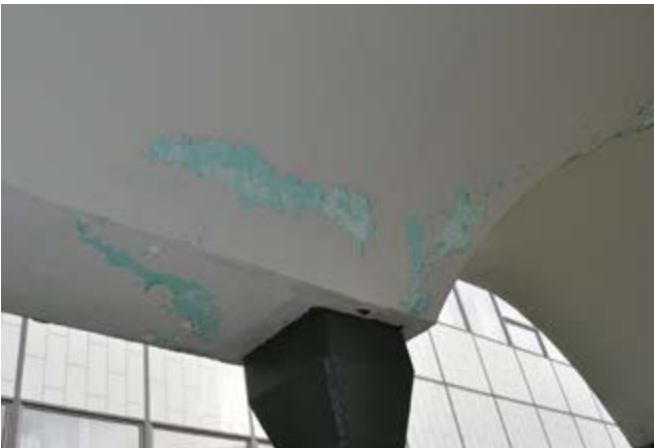
Flaking Plaster at Entrance Canopy
