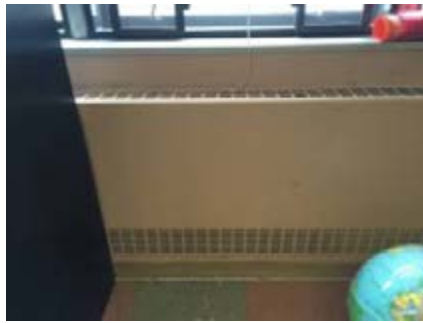
Classroom – Fin tube Radiation
