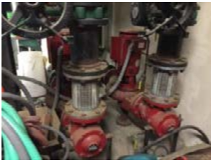
Existing Hot Water Pumps
