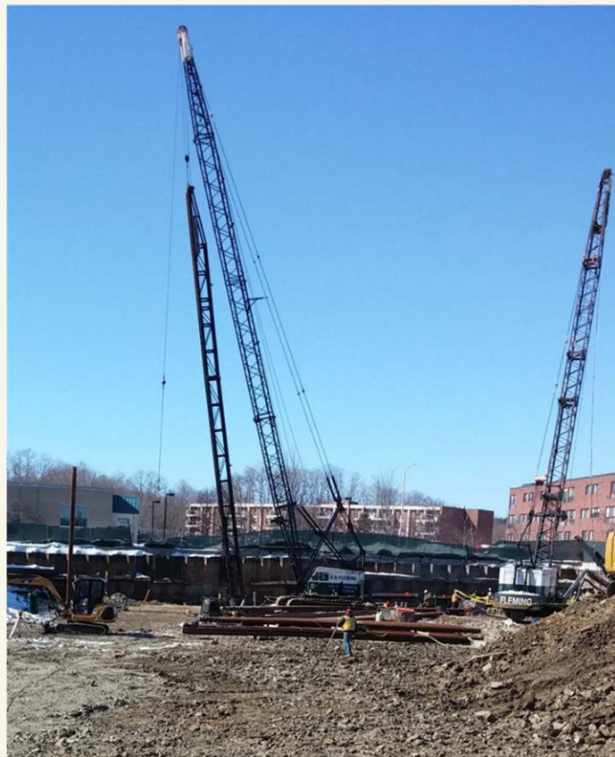
Crews use a crane to install building supports piles along the Chestnut Street side of the site.
