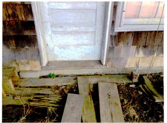
Grade at Basement Door
