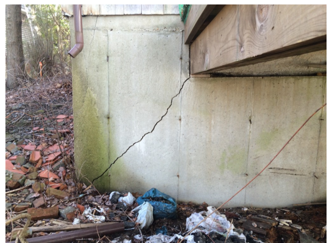
Foundation Repair Needed
