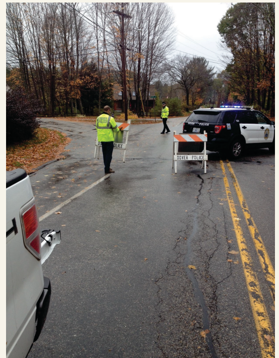
On October 28, 2016 following a fast-moving rain storm resulted in downed tree limbs and utility wires on Middle Road. Officer Lynch looks on as Officer Lazos sets up barricades to divert traffic.
