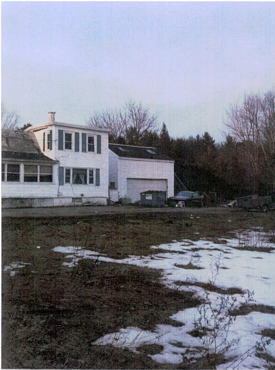
Existing Distressed Lot and Structure
