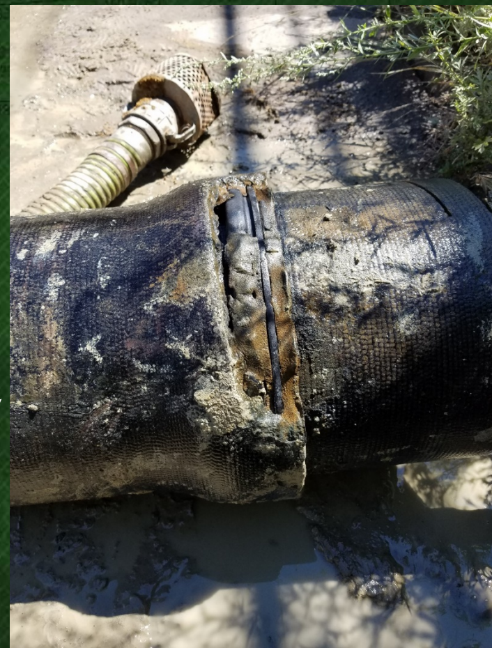
External corrosion – leak Washington Street August 2017
