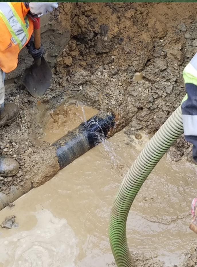
Broken cast iron main Summer Street Feb 3, 2018
