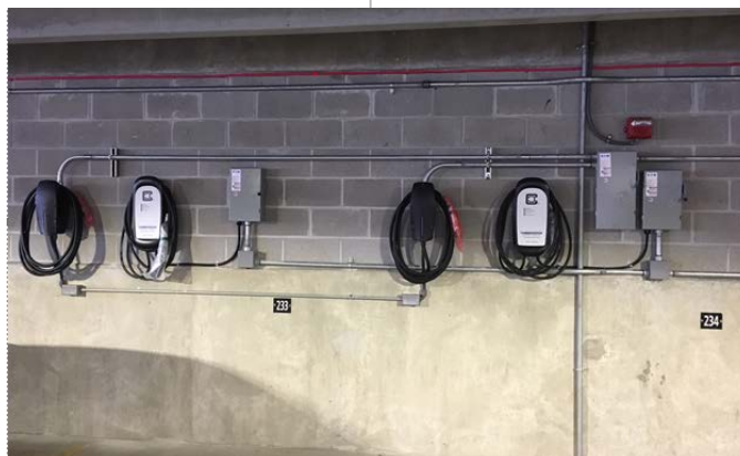
The above picture shows the wall chargers for Electric Vehicle Charging recently installed in the parking garage.
