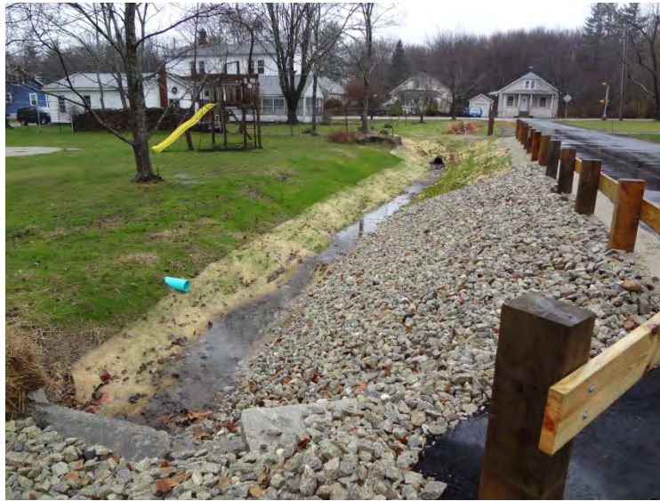
Figure 17: Snow Avenue Vegetated Swale with new pavement and guard rail installed along Snow Ave. System installed in September and October of 2011.
