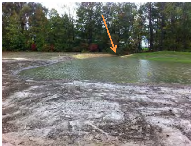
Figure 4: Crescent Avenue Vegetated Swale installed in October 2011. Arrow in picture points to the discharge point of the swale into the restored surface wetland system.
