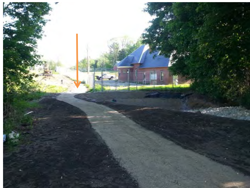
Figure 9: Roosevelt Avenue pedestrian pathway leading over stone infiltration trench (arrow) and up to Berry Brook upper watershed restoration area.
