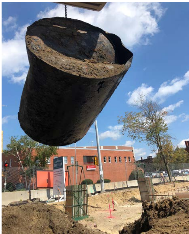
Photograph 3 - View of tank being removed from ground. Moderate to severe corrosion was noted on bottom of tank. (StoneHill, September 6, 2018)
