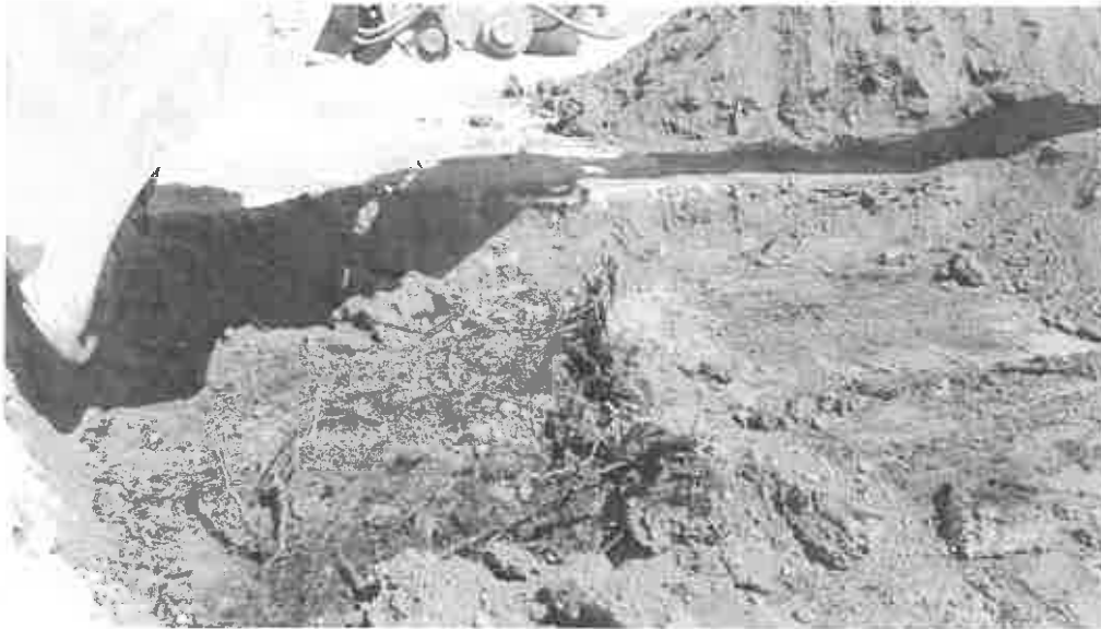
Organic matter approximately 6 inches below top of clay subgrade.
