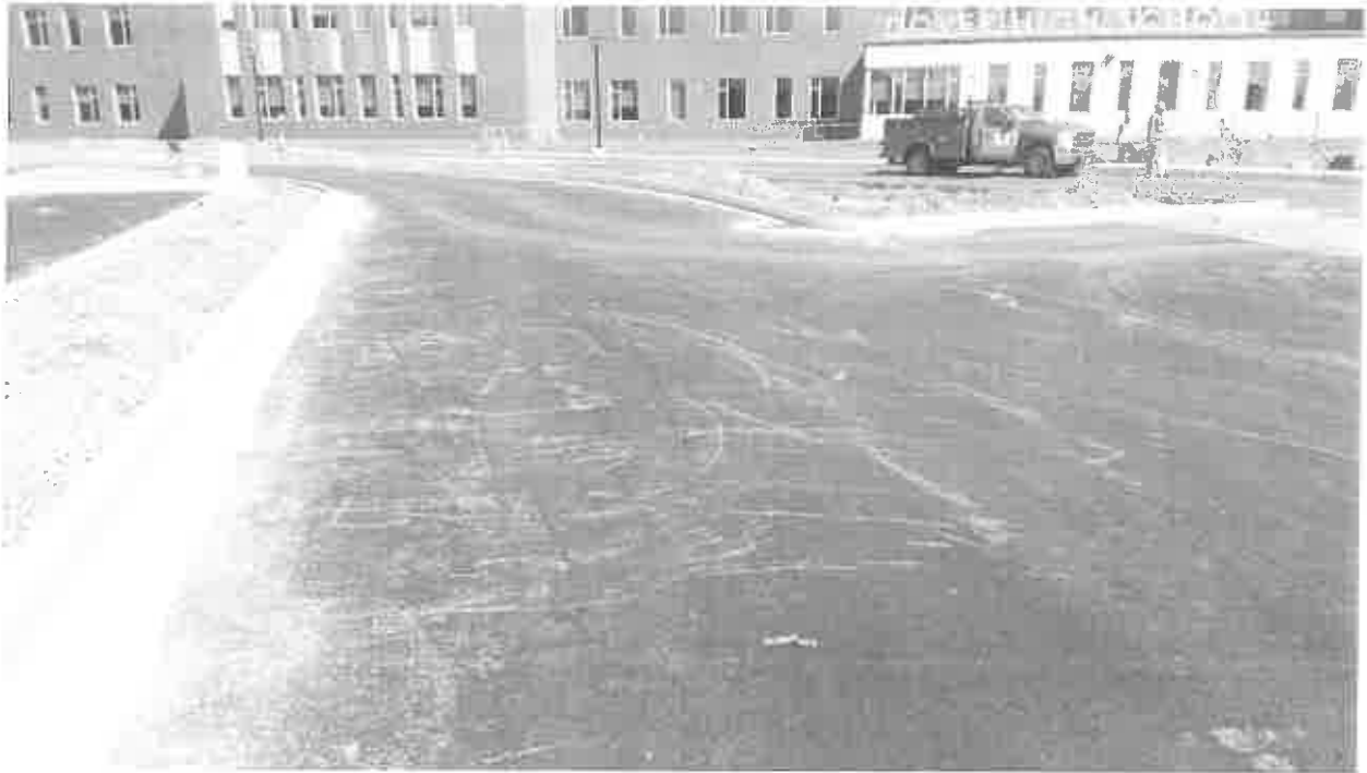
Areas of observed pavement distress in northern portion of main parking lot
