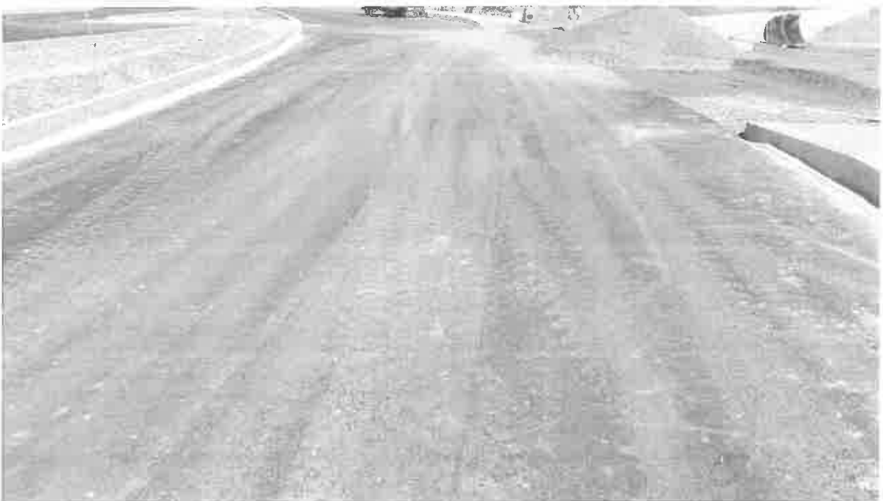
Area of observed pavement distress east of entry plaza in main drop off isle
