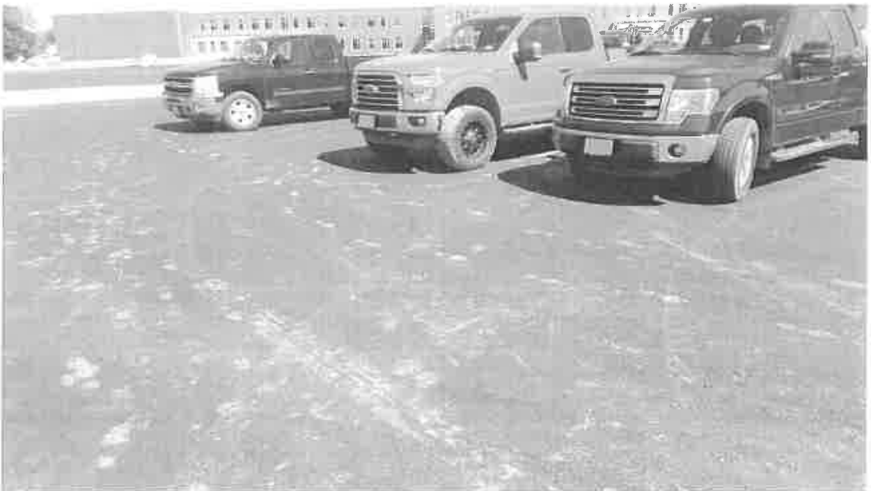
Areas of observed pavement distress in southeast portion of main parking lot
