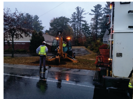
Above, Unitil crews locate the most appropriate location to shut off the gas leak, occurring over 100' away at the rear of the Office Park shown in the background.
