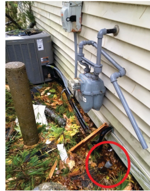
Severed gas line circled in red above.
