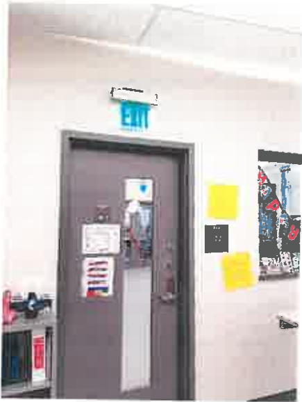
Broken pull station at door A-06
